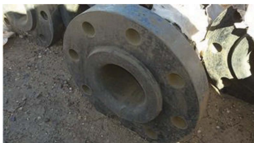
Figure 12. CHF reticulation system pipework.
