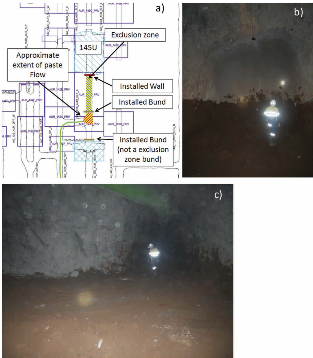
Figure 9. Paste 145U overflow showing a) level plan with approximation of location of bunds, b) paste staining at the shotcrete wall location, and c) paste staining along the drive.
