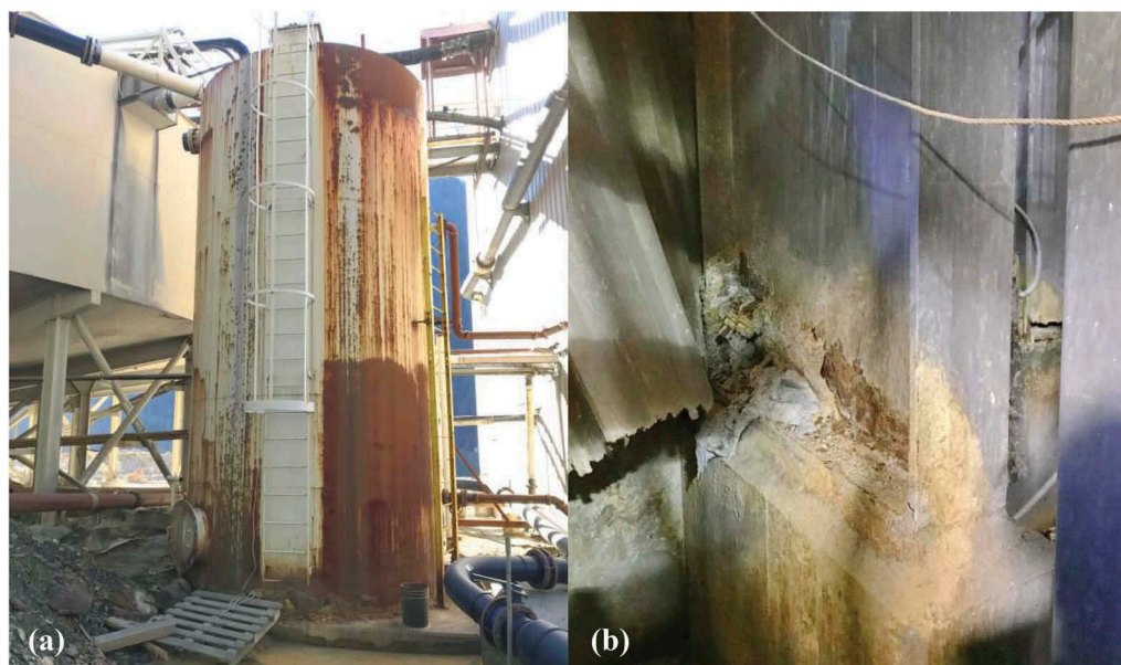
Figure 7. Examples of existing equipment corroded from contact with tailings (a) Process water tank and (b) Building column.
