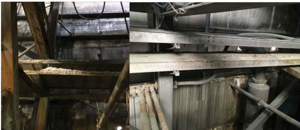
Figure 10. Cable tray's full and corroded/full of tailings.
