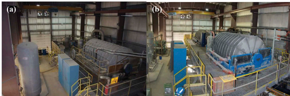
Figure 6. Comparison between (a) Existing filter level layout and (b) Retrofit filter level layout.
