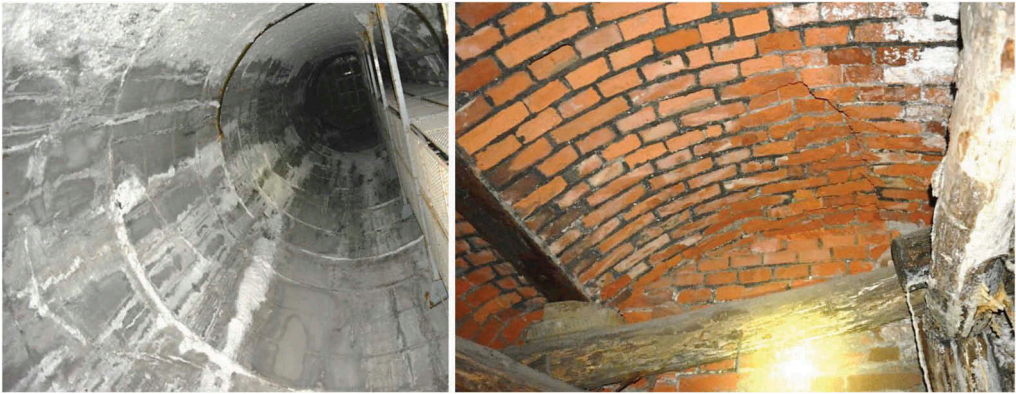
Figure 6. Damage to the shaft lining and shaft bottom supports occurring in the vicinity of the level IV.
