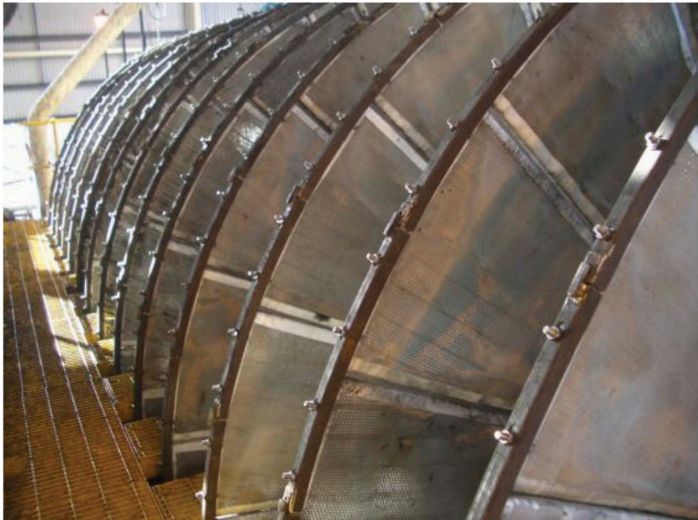
Figure 7. Revamped filter with improved access along the filter by permanent walkways.
