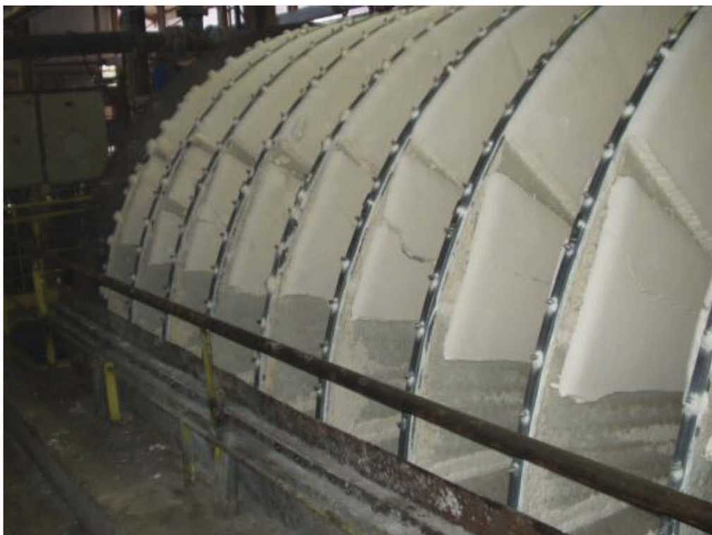
Figure 3. Complete cake discharge of a type A disc filter after revamping with “large package” modifications.
