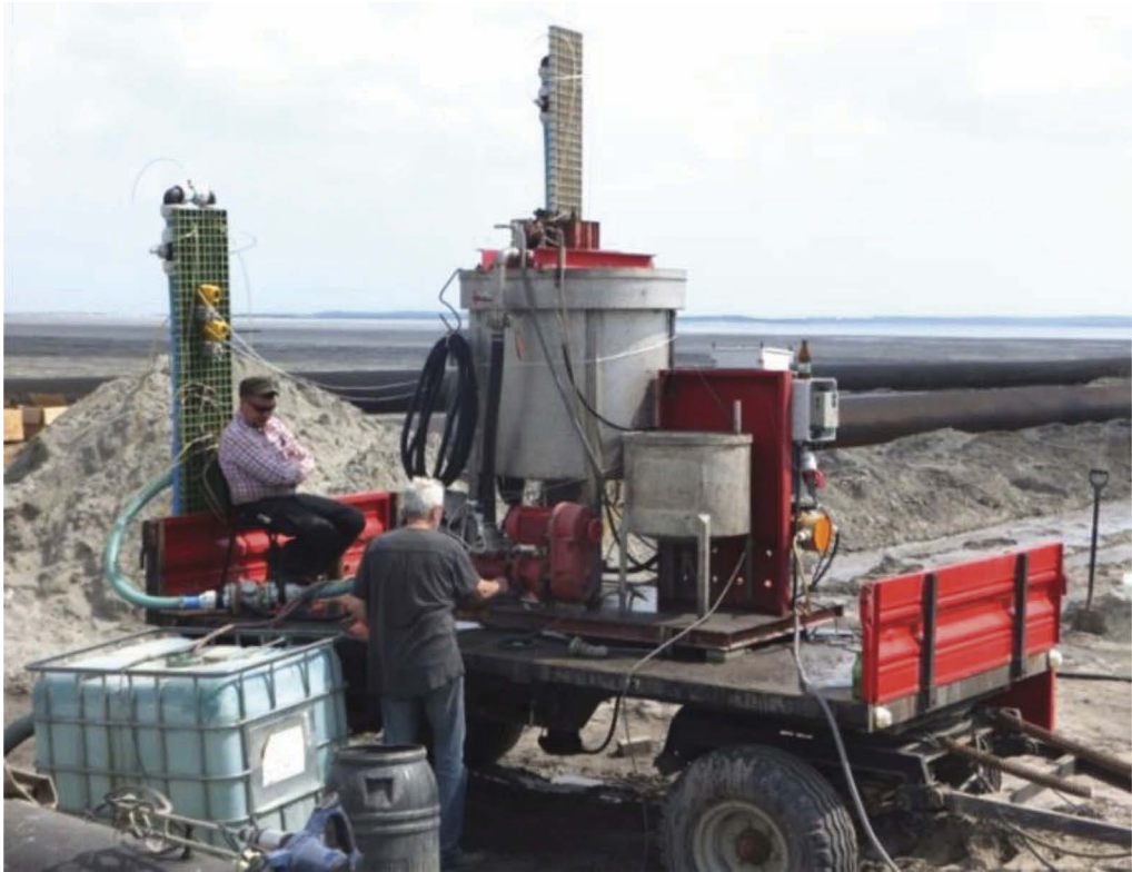
Figure 1. Mobile Thickening Unit during measurements.
