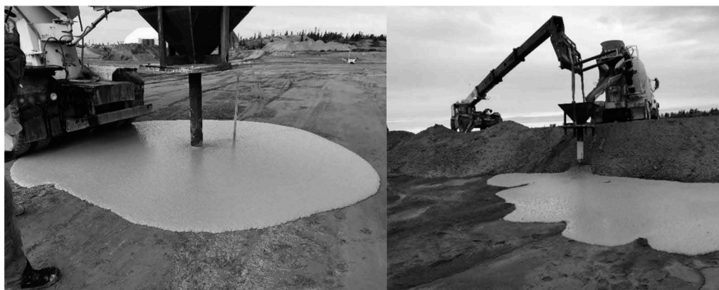
Figure 5. Full scale SCC trial batching on the surface. Source: MineFill Services project database.
