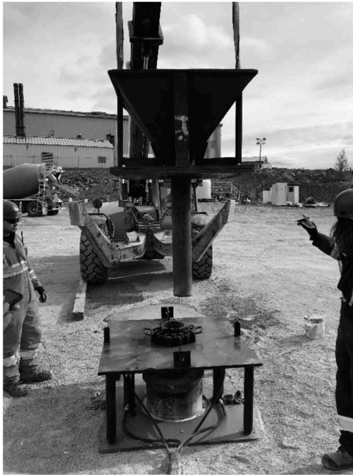
Figure 6. Hydraulic jacks for raising the tremie pipes. Source: MineFill Services project database.
