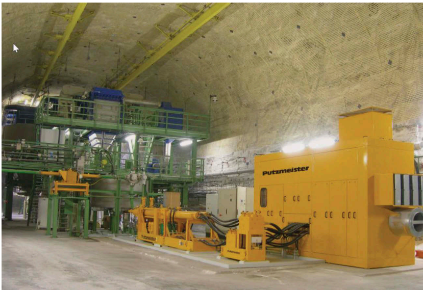
Figure 13. Underground Backfill Plant at Kali & Salz.
