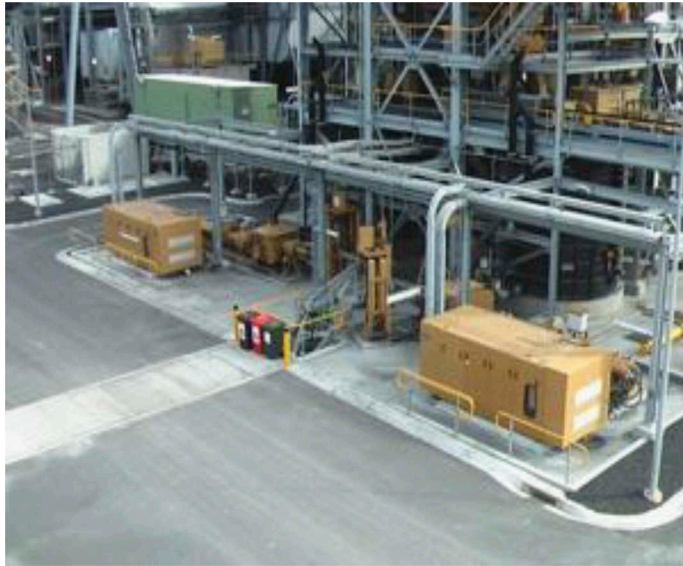
Figure 14. Fly- and bottomash pumping station at Kogan Creek.
