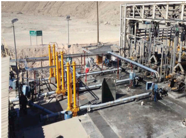
Figure 15. Tailings pumping plant at Coemin with VPD.
