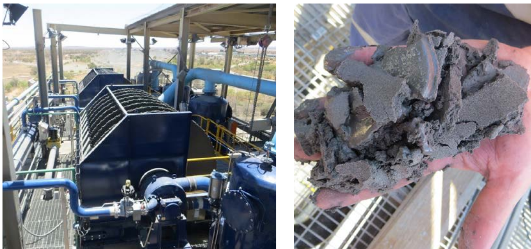
Figure 4. Two Boozer disc filter ME8 (141 m 2 filter area each) for zinc tailings dewatering in the filter building (left); discharged filter cake (right)
