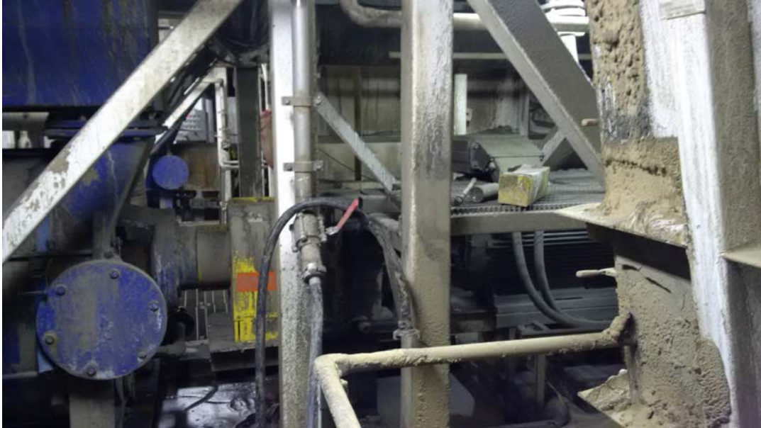
Figure 2. Vacuum pump contained within a ‘modular’ structure which limits maintenance and operations access
