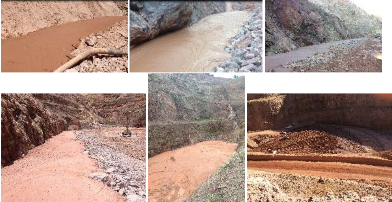
Figure 7. Progressive deployment of fill into mined out open pit - continued. Upper left and middle: Paste pouring against hanging wall fault to prevent water ingress. Upper right and lower left: Cemented paste allowed to dry. Lower middle: Additional layers of cemented paste poured and allowed to dry. Lower right: Stacking of filtered tailings. Courtesy of Agnico Eagle Mines Limited.
