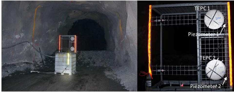
Figure 6. In Situ instruments installed in the 721 XC
