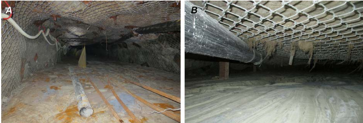
Figure 3. Gap between consecutive backfill levels: (a) 1-m (3-ft) gap above the 5550L-11E stope and (b) 0.3-m (1-ft) gap above the 6350L-15W stope
